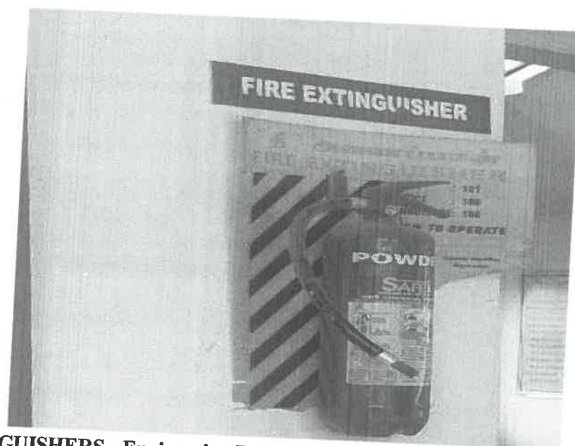
FIRE EXTINGUISHERS - Main Building - First Floor
